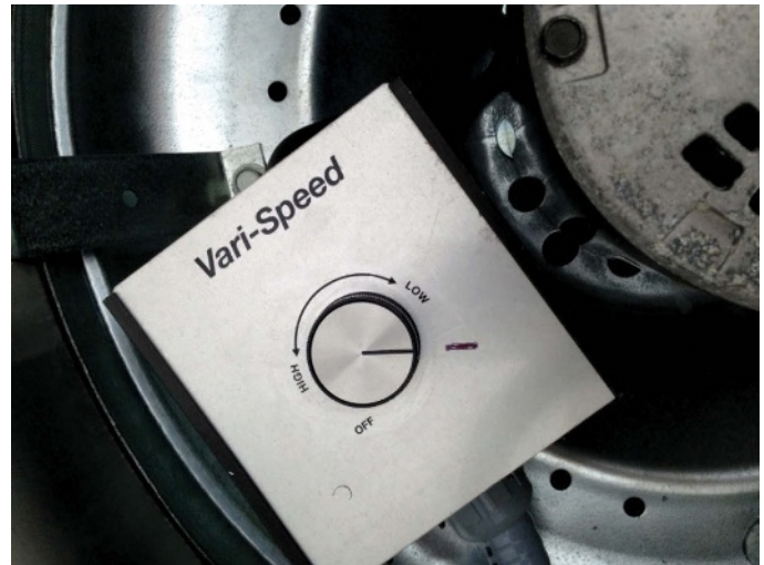
Figure 2. Greenheck CUE 121 Fan - Fan motor with adjustable speed controller.
